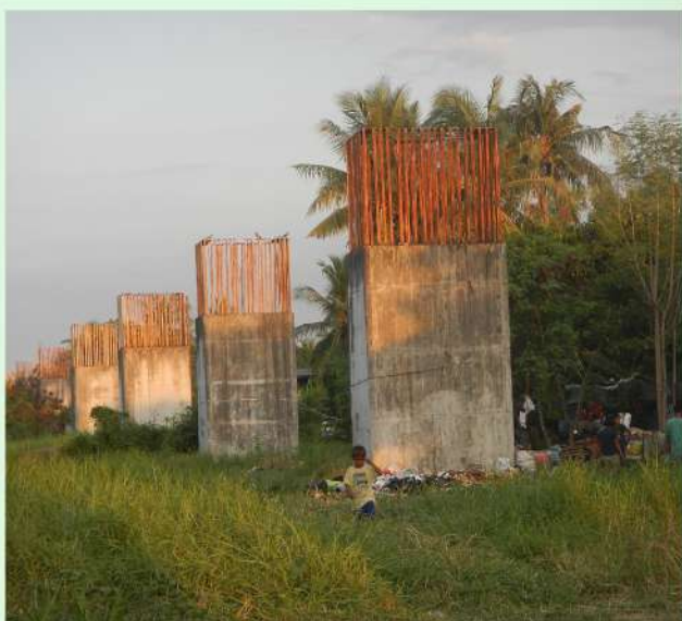
Remains of the failed North Rail Project by NBN-ZTE in Bulacan. Photo from Wikimedia Commons, Public Domain.
